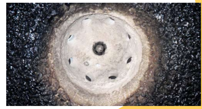
Roof burner within combustion chamber, 1,000 kg/h fuel oil TWL Technische Werke Ludwigshafen AG
