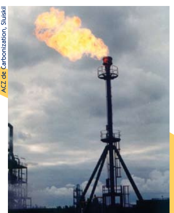
Flare for coke oven gas
